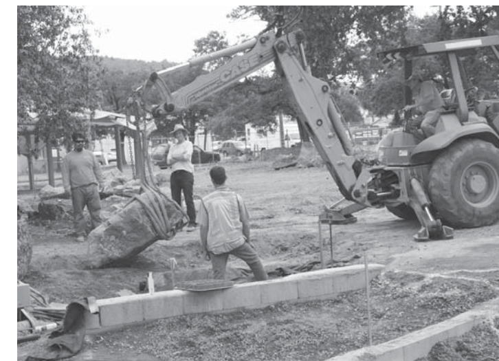
Workers from Siri Grading and Paving and Ann Baker, lead project designer, moving rocks into place for The Salmon Stream.
